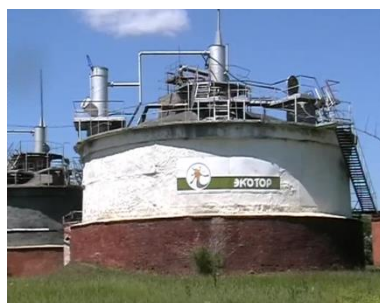
Engels city WWTP, in operation (Russia, 2002)
