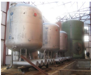
Zhitomir city WWTP, commissioning (Ukraine, 2007)
