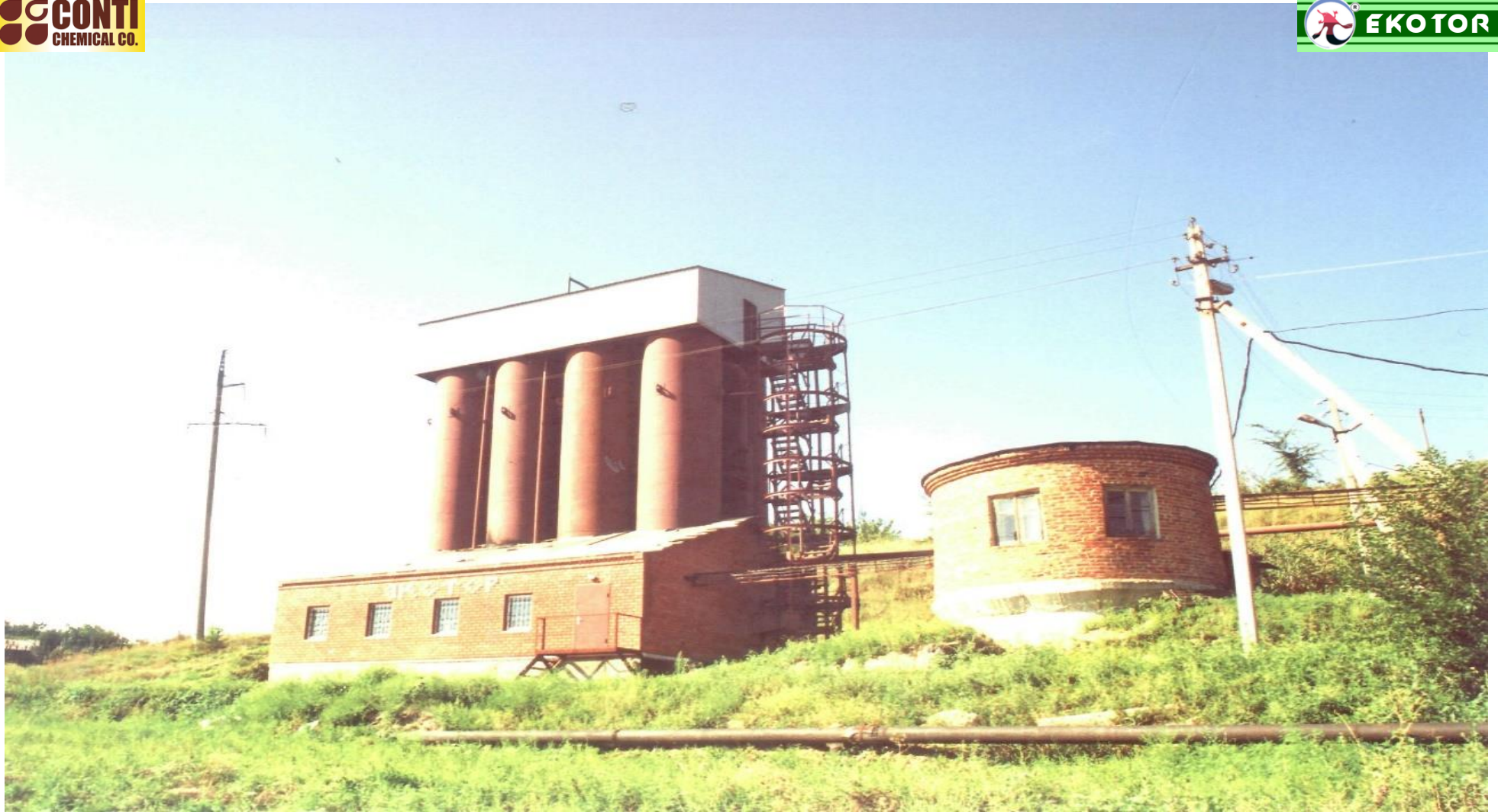
Local WWTP of Tambov alcohol refinery. Capacity 2500 m 3 per day. 2002, Tambov, Russia
