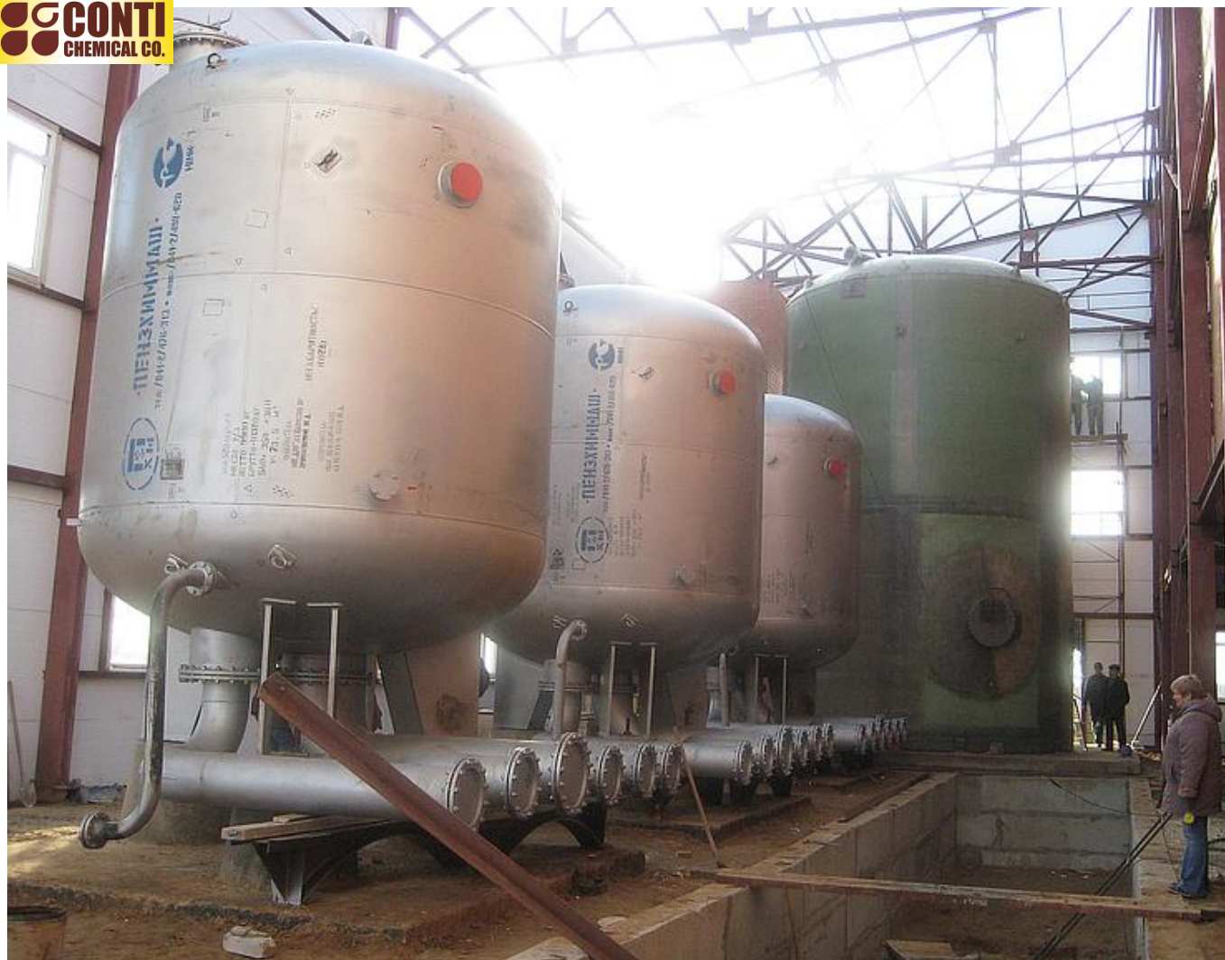
Sludge treatment at Kolomna city WWTP. Sewage capacity 90 thous. m 3 per day. 2014, Moscow region, Russia
